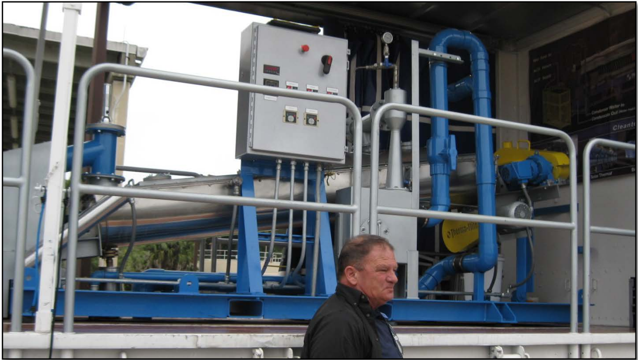
View from the other side of Indirect Drying System showing Dryer behind the Control Panel
